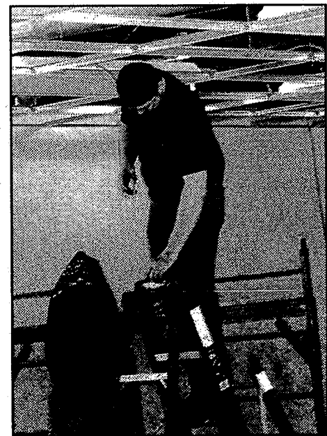
Brian Abbott works on wiring above the drop ceiling. Photo by Trevor Keiser.
