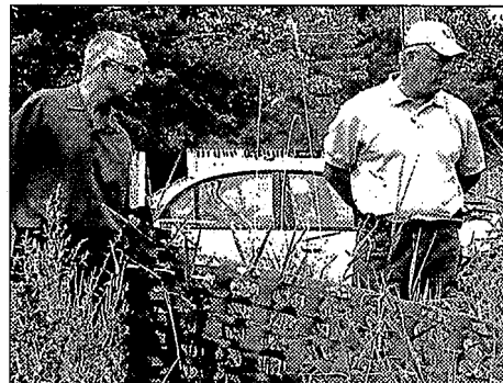
Springfield Township Supervisor Mike Trout and Mike Forst, property manager, check a compromised septic system off Broadway in Davisburg. Photo by Phil Custodio
