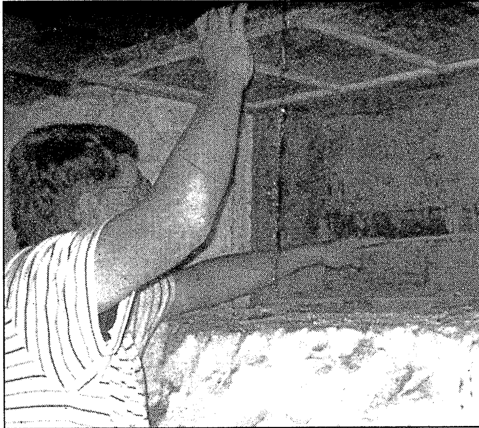
Dean Farner checks a basement window for leaks. Photo by Wendi Reardon
