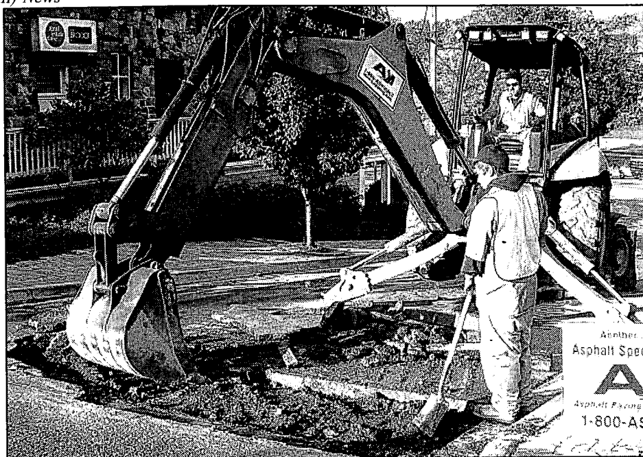
Workers use a backhoe to dig up the old asphalt on Depot Road. Photo by Phil Custodio
