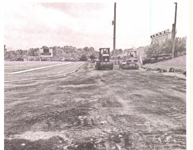
NOVI SCHOOLS Construction has started for a new eight-lane track at Novi High School.
