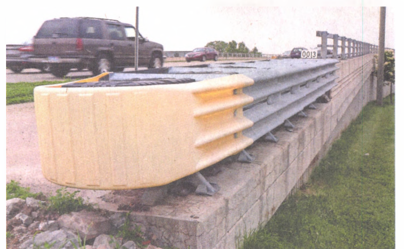
Oakland County will soon be doing maintenance work on the Grand River Avenue bridge, just west of Novi Road. The bridge was rebuilt in 2004.
