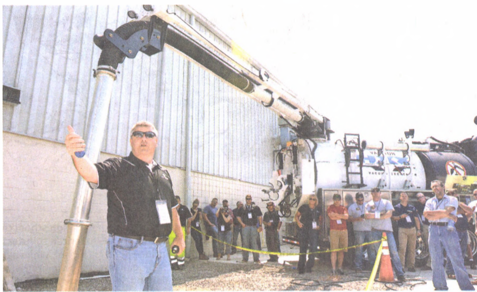
JOHN HEIDER | STAFF PHOTOGRAPHER Mike Suitor instructs industry representatives on how to use a Doheny vacuum truck for hydro-excavating during the Northville business' recent open house and seminar. Hundreds of workers from the U.S. and Canada stopped by to see the latest gear Doheny has at its Northville shop.
