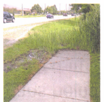
The city of Novi will be continuing the sidewalk on the east side of Novi Road between Nick Lidstrom Drive and 10 Mile Road.
