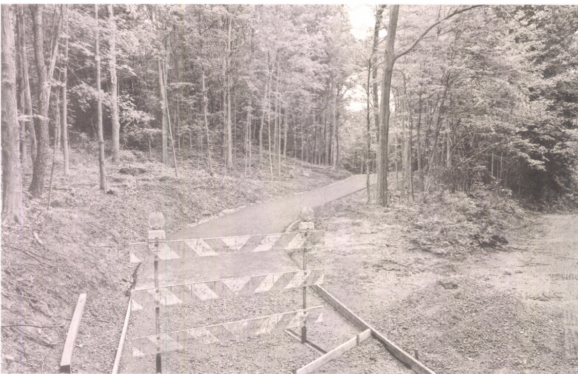
Work continues July 8 on the paved walking and biking path through Maybury State Park. The path, which begins near Eight Mile and Beck roads, will loop through the park. This terminus is near the pond on the southeast side of the park.
