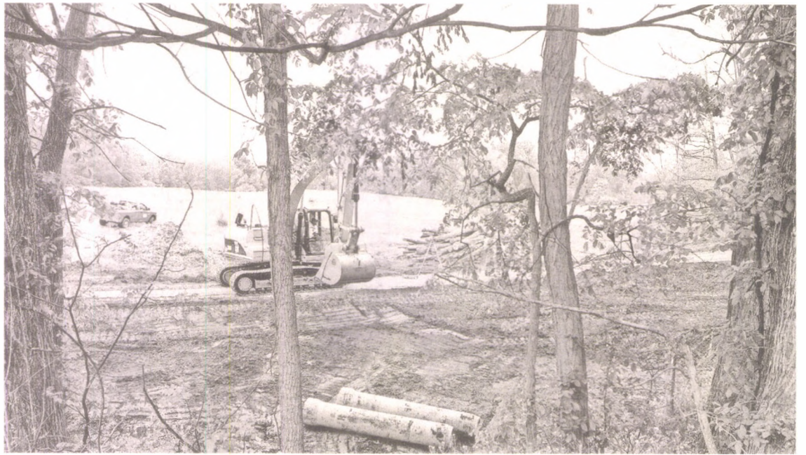
Work continued on May 26 for the pedestrian path near Maybury State Park's northeast corner at Eight Mile and Beck roads. When completed, the path will give safer, better access to the park for visitors entering on foot. The project is jointly funded and organized by Wayne County, Northville and Northville Township.
