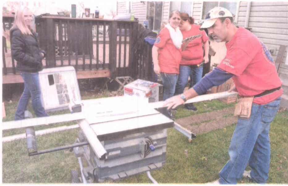
Kim Strange (left) watches as Lowe's employee Todd Amprim (right) cuts a piece of flooring for the Strange home in South Lyon recently during Lowe's Local Heroes effort. Lowe's and its employees were helping to renovate and make the house more accessible for their daughter Breanna, who has dystonia.
