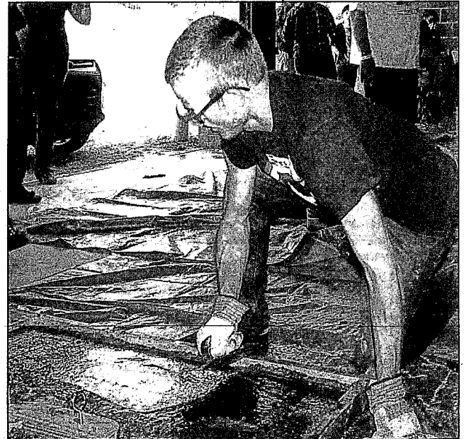
James Rice, senior at Michigan State University and president of the MSU Engineers without Borders chapter, works on a cement cover. Photos by Phil Custodio
