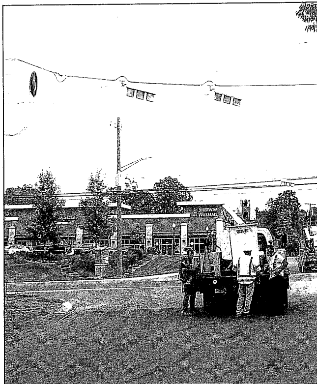
NEW LIGHT: Crews install a new traffic light at the intersection of Sashabaw and Flemings Lake Road, a dirt road. The $150,000 light was approved in October 2012 and funded through Tri-Party funding, the Road Commission for Oakland County, Corridor Improvement Authority and the County Board of Commissioners. The light was installed, Oct. 2, in a location where several accidents, including one death, had occurred.
