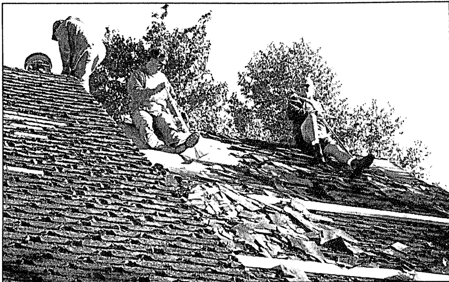
Bank of America volunteers reroof a home in Independence Township. Photo provided
