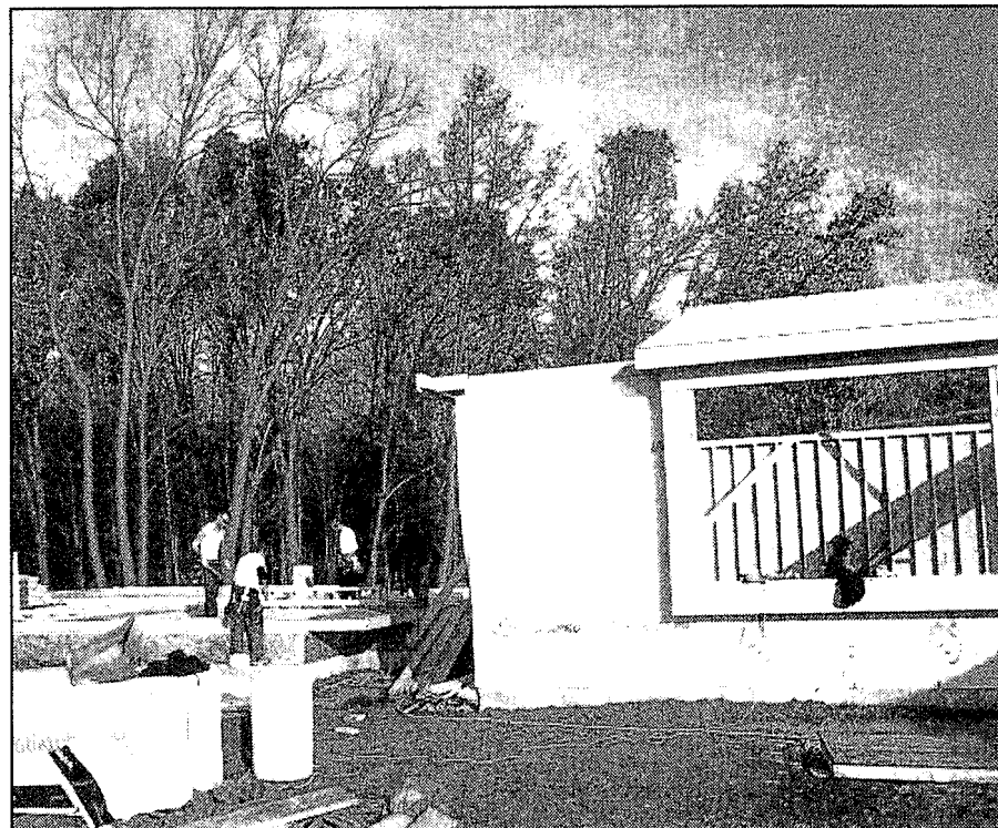
A house under construction on Bitterbush Drive, in the northwest section of the township. Photo by Joette Kunse
