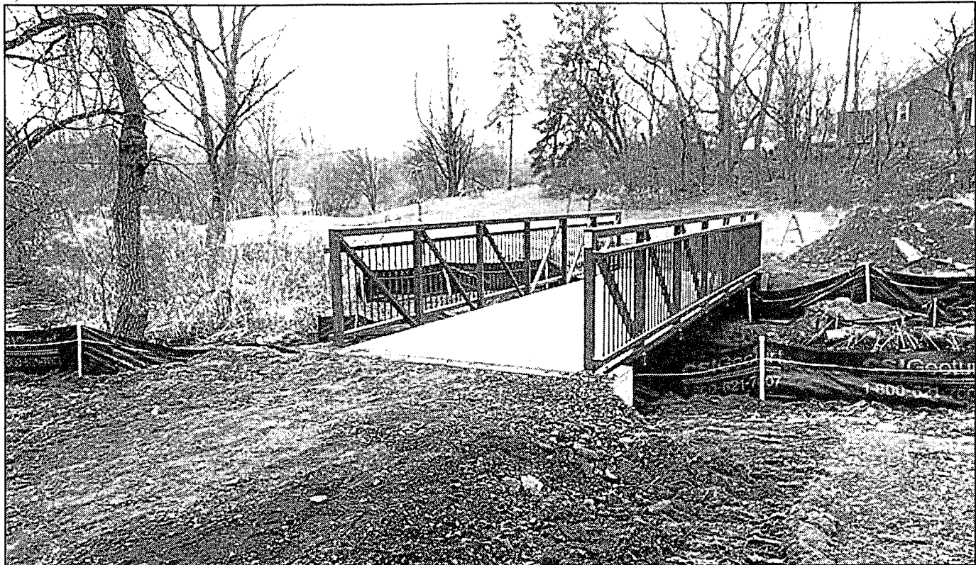
The new bridge in Depot Park will get more work in the spring, but is ready for walkers to cross. Photo provided
