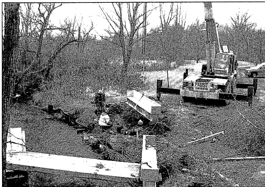
Workers from Faust Corporation install footings for the new bridge earlier this month. Photo by Phil Custodio
