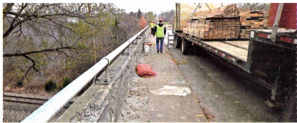
JOHN HEIDER STAFF PHOTOGRAPHER Crews from C.A. Hill Co. work on the Eight Mile bridge over the CSX railway tracks.
