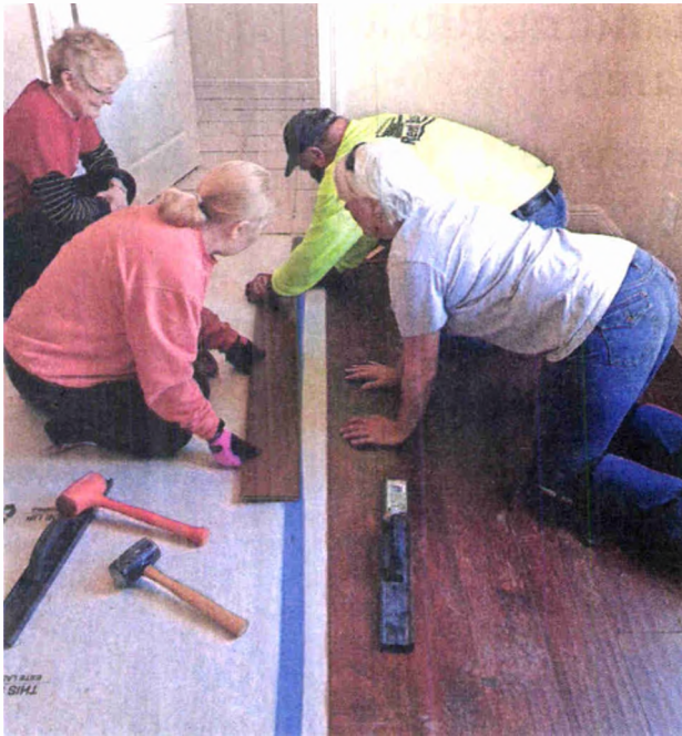
Church volunteers install flooring in one of the two houses in which they worked during their trip.
