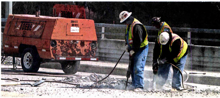
The eastbound ramp over I-275 at Seven Mile is already closed as workers begin removing and replacing its road surface. The effort is part of the reconstruction efforts on the major highway that lies between Northville, Novi and Livonia and Farmington Hills.
