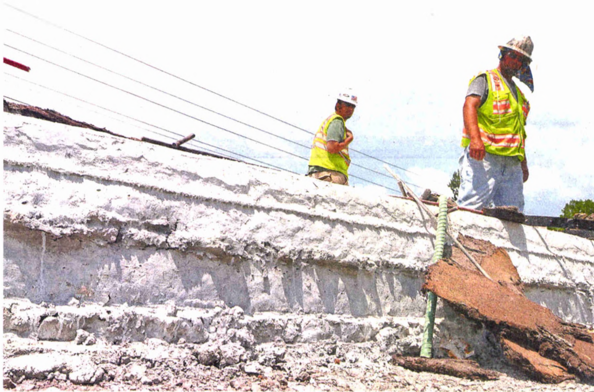
A recently poured section of concrete shows its one-foot depth on I-275's southbound lanes. Crews subcontracted by MDOT have been working on the highway since early May.
