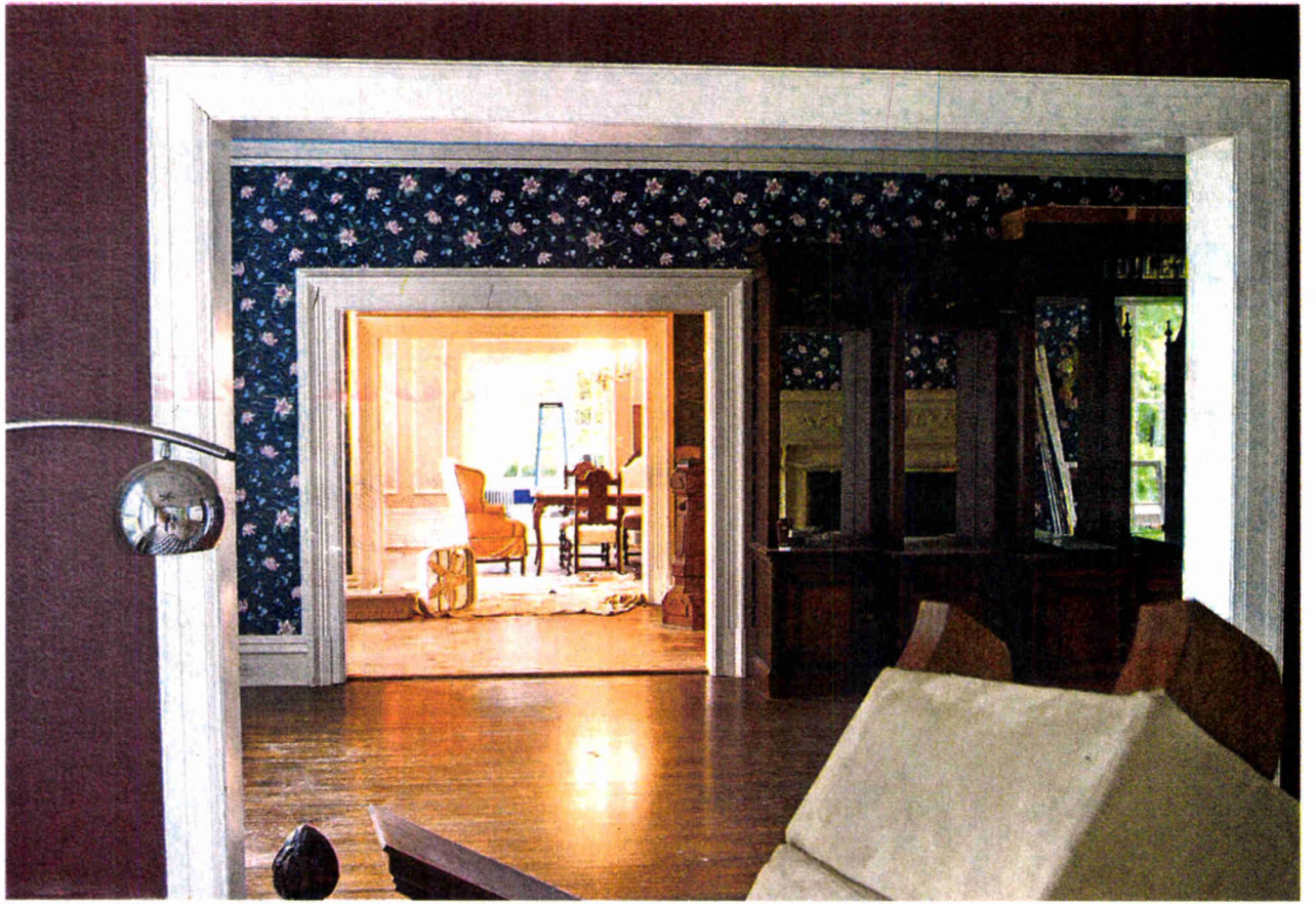
While the house is in disarray with work being done throughout, a view from one end to the other is still visible.
