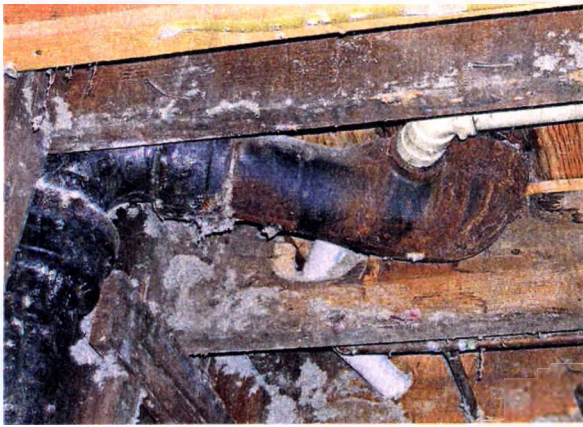
A notched joist.
