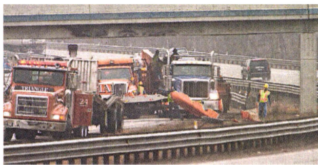
Workers remove debris from the truck that hit the old Eight Mile Road overpass at U.S. 23 in Green Oak Township. The overpass was demolished and rebuilt. Now a totally new overpass with roundabouts is open to traffic.
