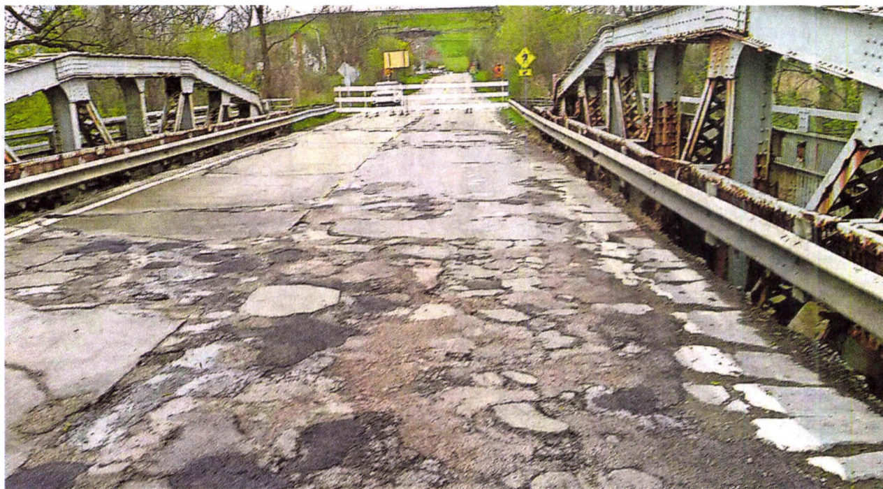
An engineering firm has recommended this Lilley Road bridge in Canton be replaced.
