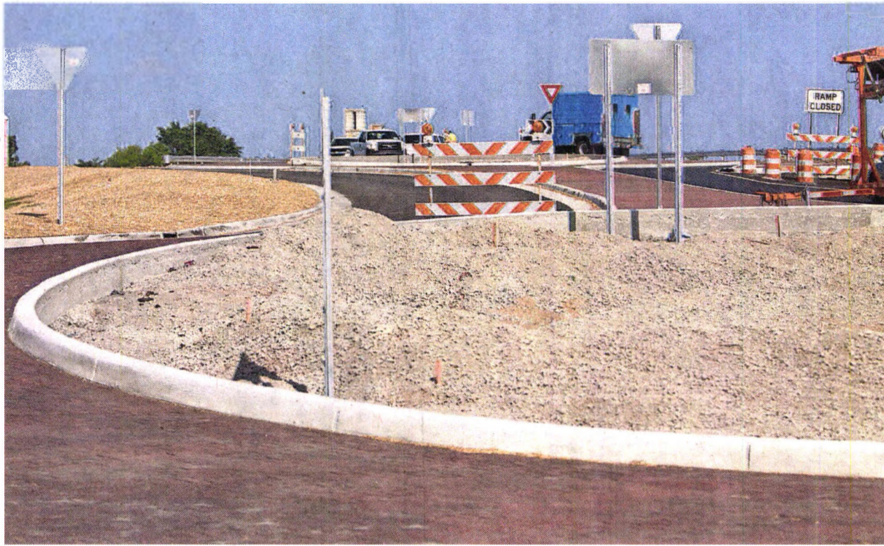
A triple roundabout traversing U.S. 23 at Eight Mile Road in Green Oak Township opened to traffic June 14.
