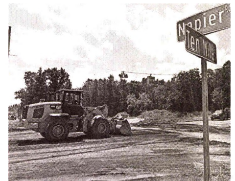
JOHN HEIDER | HOMETOWNLIFE.COM Work continues at the intersection of 10 Mile and Napier in Lyon Township.
