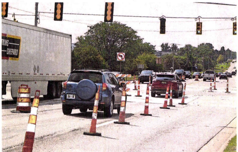
The Road Commission for Oakland County is working on a concrete road surface reconstruction at the corner of Haggerty and 10 Mile until early September. The county will intermittently close right-turn lanes as workers replace the road surface. Some delays in the area will occur.
