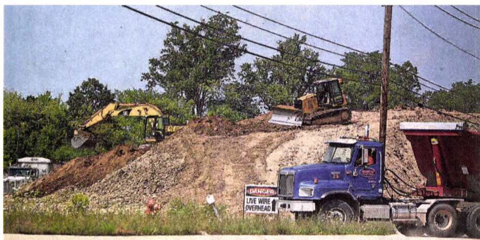
Work continues Aug. 16 on the prep stage of Novi's Brooktown development at the southwest corner Grand River and Meadowbrook. The 26-acre mixed commercial and residential development sat idle for many years, but infrastructure work, including roads, water and sewer and moving a large pile of soil, seen at right, has begun.
