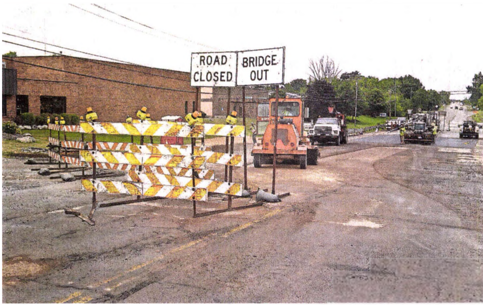
JOHN HEIDER | HOMETOWNLIFE.COM Crews continue to wrap up a resurfacing project on Meadowbrook, north of Grand River, Aug. 28. Meadowbrook was closed to northbound traffic until the week before and then was entirely closed near the I-96 overpass as crews finished working on the road's surface just south of the overpass. Meadowbrook was to completely reopen later that week.
