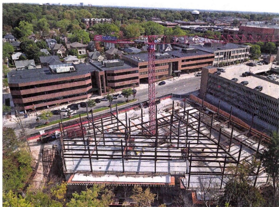
An overhead view of Brookside Terrace taken by a drone. The project broke ground in early October. ALDEN DEVELOPMENT GROUP
