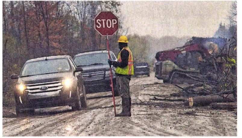
Crews are getting Napier Road between Nine and 10 Mile ready for upcoming paving. The road will close beginning Nov. 10 and is expected to reopen Jan. 5. BILL BRESLER | HOMETOWNLIFE.COM
