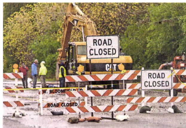
Roads had to be closed as crews worked to repair the water main break. BILL BRESLER | HOMETOWNLIFE.COM
