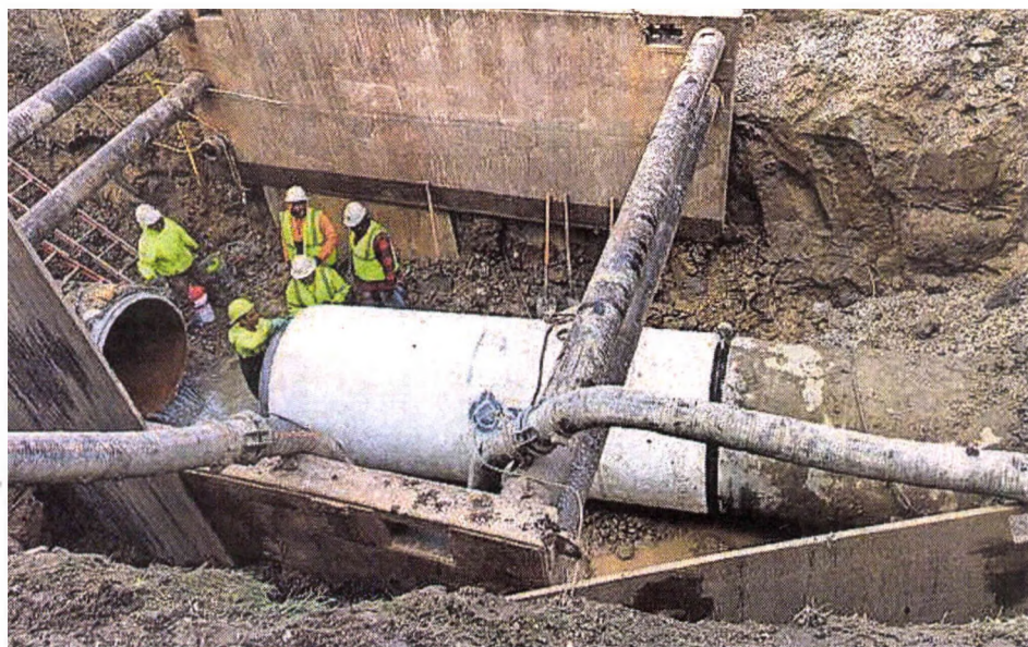
Crews had to work to repair the break. GREAT LAKES WATER AUTHORITY
