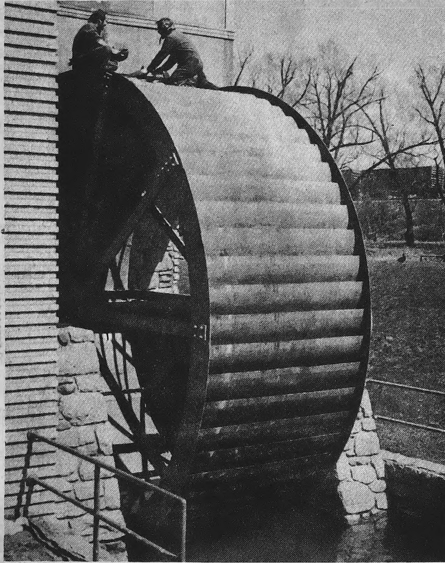
ROLLING AGAIN —Mickey Martin and Ralph Silvers of the Ford Valve Plant's maintenance crew in Northville are shown repairing the famous water wheel landmark. This week it's turning again. What's more, it's been given a patriotic facelift — red, white and blue stars and stripes. It's all part of an effort encouraged by Mike Fras, superintendent of the local Ford plant, and Bill Beauchamp, the maintenance chief, to spruce up the grounds. (See "Speaking for The Record"—page 8-A.)
