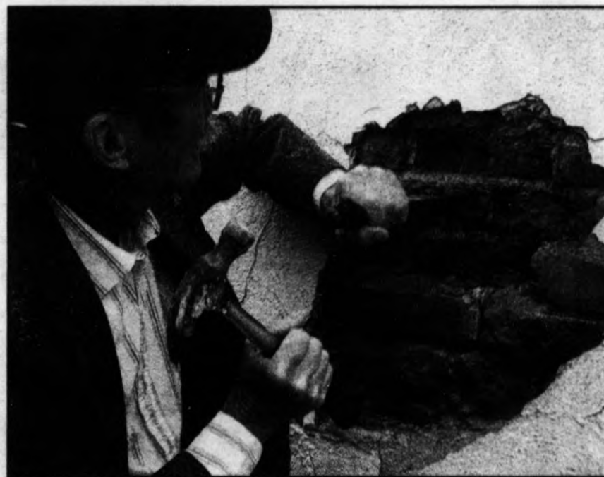
RESTORATION: Timothy Mack, general contractor, hammers out a sample of brickwork from 5 S. Main Street in order to match it during restoration. See page 4 for more. Photo by Phil Custodio
