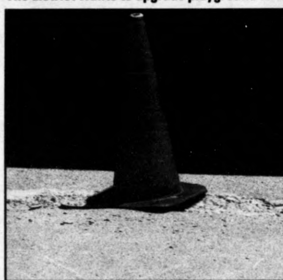
A cone marks an unsafe walkway.
