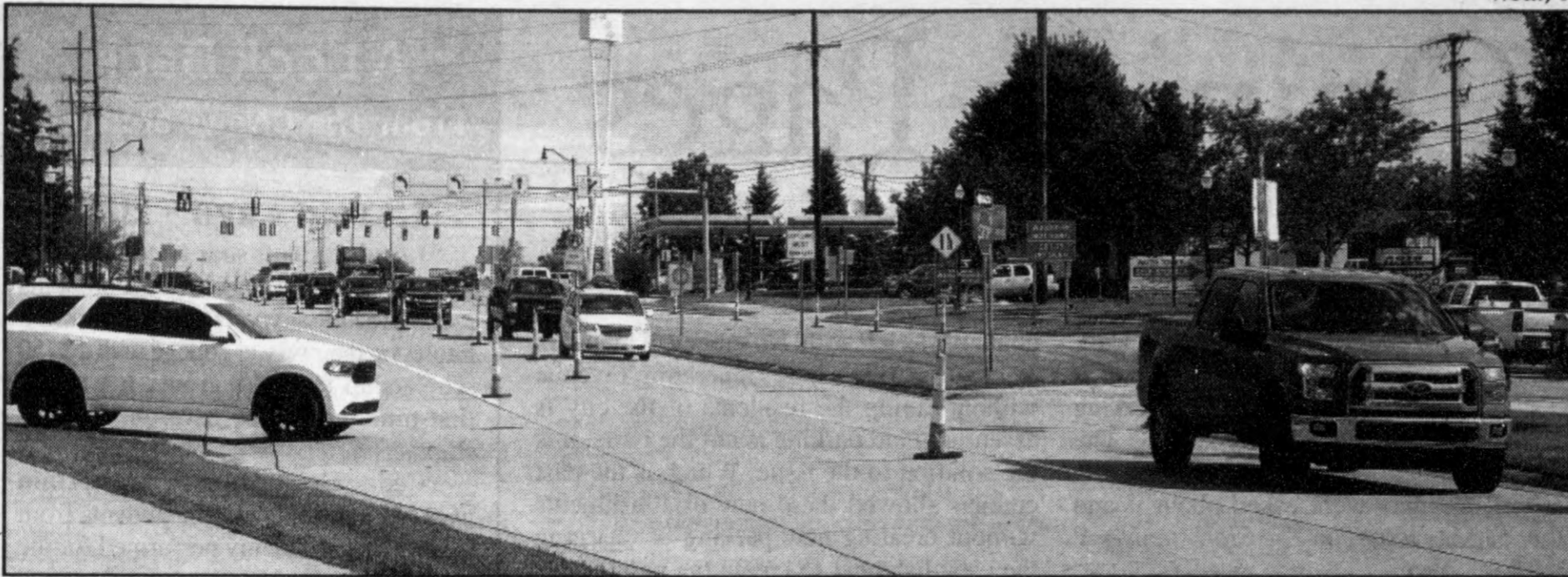
Concrete slab replacement work on Sashabaw Road is expected to continue through the end of the month. Cipparrone Contracting Inc. is performing the work on Sashabaw from Maybee Road to Waldon Road in Independence Township. Photo by Phil Custodio
