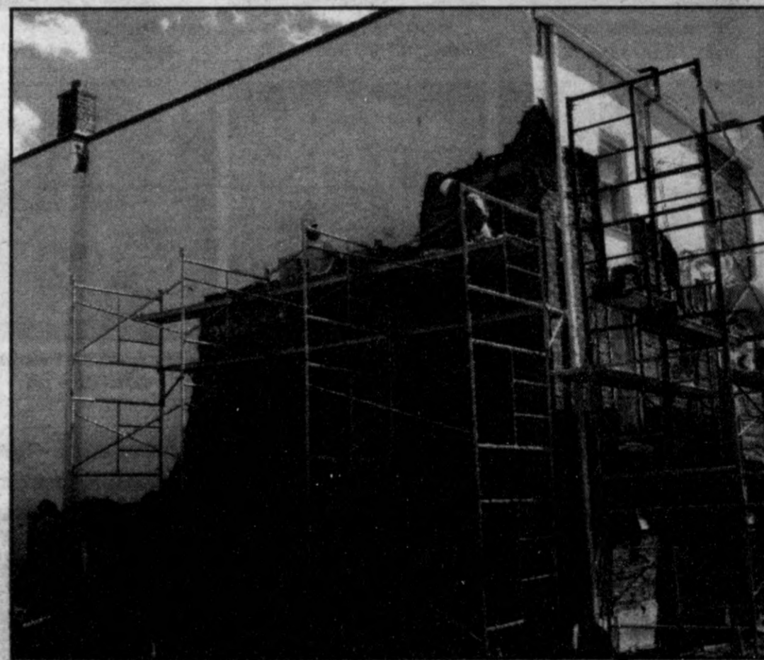
Chris Blaine of Top Hat Masonry Repair, at right, leads rebricking work on 5 S. Main Street. Photo by Phil Custodio
