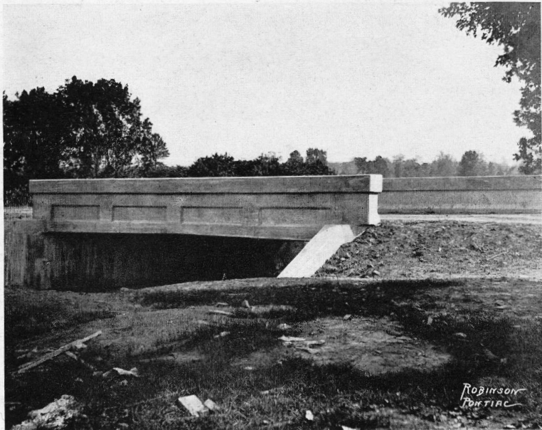
A fine specimen of reinforced concrete girder construction. 12-Mile Road, Royal Oak Twp.
