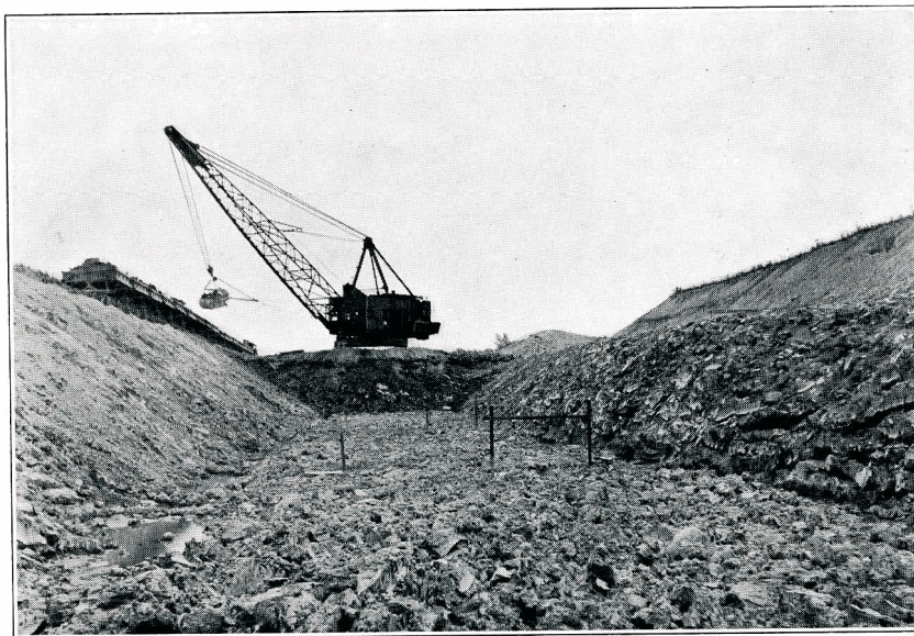
Thousands of Cubic Yards of Earth Work Removed to Make Rapid Transit Possible
