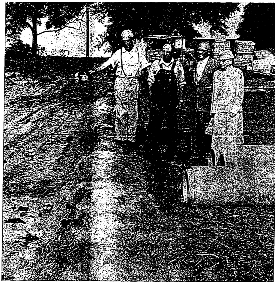
NORTHVILLE township will soon have its first subdivision with sanitary sewers. Connection to the Middle Rouge Interceptor is already underway on Bradner road through property owned by Russell Rinehart, shown above (left) meeting to the north of the connection. Rinehart, 1577 Bradner, donated an easement to allow sewer facilities for a proposed 275-home development by the Gordon and Scheurman company of Detroit. Will Rinehart are: (l. to r.) Howard Bowring, owner of a section of the land sold for development, D. J. Siark, township clerk and realtor handling the transaction, and Mrs. Mollie Lawrence, township supervisor.
